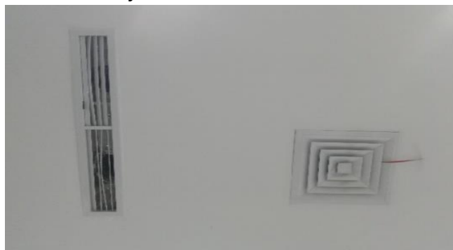
Figure 6: Central Air Conditioner (AC)
